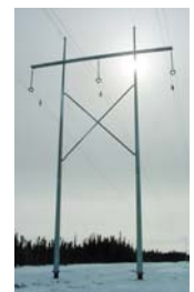
Typical 240-kV Structure
