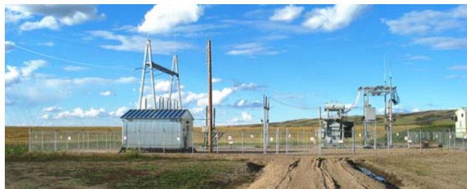
Existing Ribstone substation: a typical substation at a pipeline pump station in southern Alberta.
