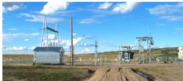
A typical substation at a pipeline pump station.
