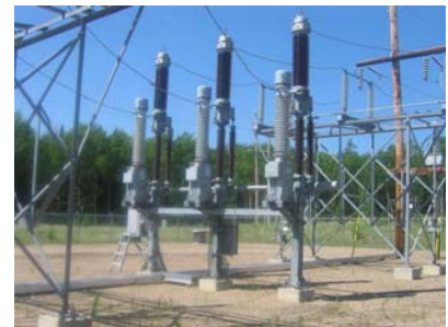
Typical 144 kV Circuit Breaker
